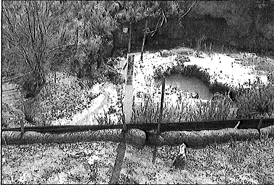
Figure 1: View of leak site from the east bank.
